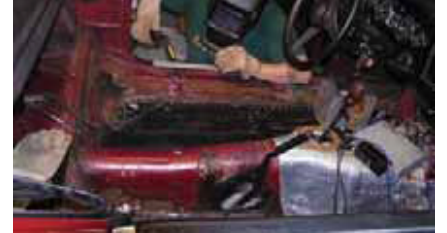
16. Spot-weld the new panel in place. (Always have a fire extinguisher on hand—better to have it and not need it than the other way around.)
