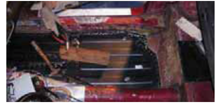
15. We used a heavy weight to keep the pan flat and in position while welding.
